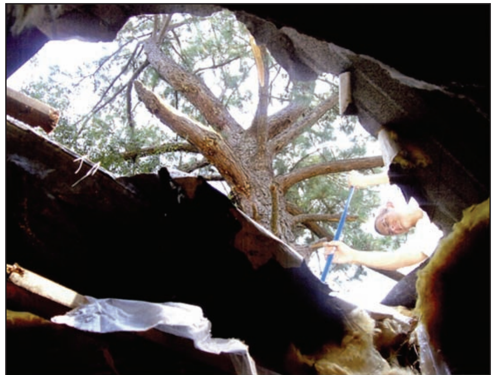
Franklin Dangerfield's home after the storm: Mobile home park's owner had been warned that damaged tree posed a danger to the homes below. Submitted photo
